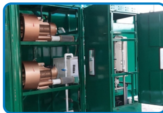
SEWAGE TREATMENT PLANT(STP)
